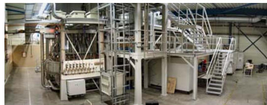
Figure 2: RGS production machine installation at RGS Development B.V.
